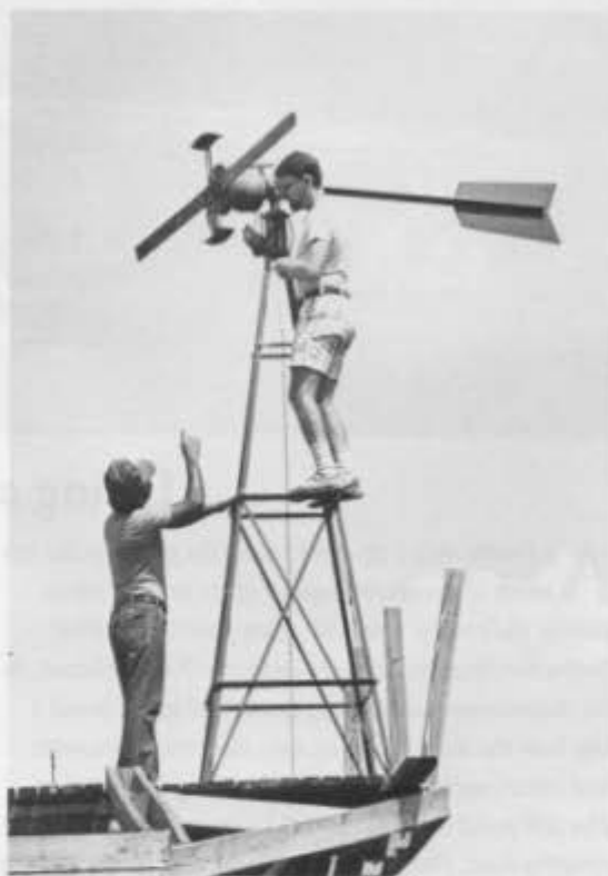
Students in the Environmental Demonstration Center on South Campus install a windmill to generate electricity.
