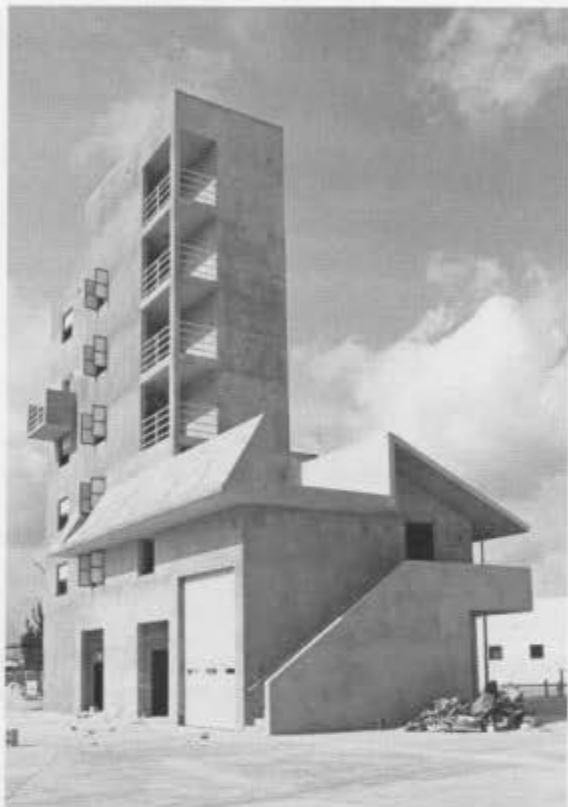
Construction was underway in November 1983 on the $2.6 million Southeast Florida Academy of Fire Science. It opened on a one-acre site at the corner of the North Campus.
